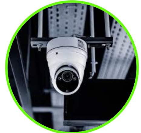
SASB-CCTV installation for security and quality improvements
